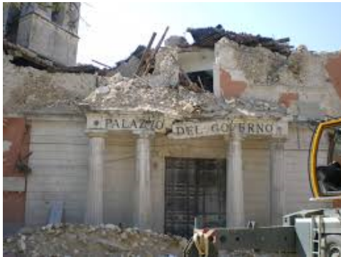
Damage after earthquake in L'aquila
